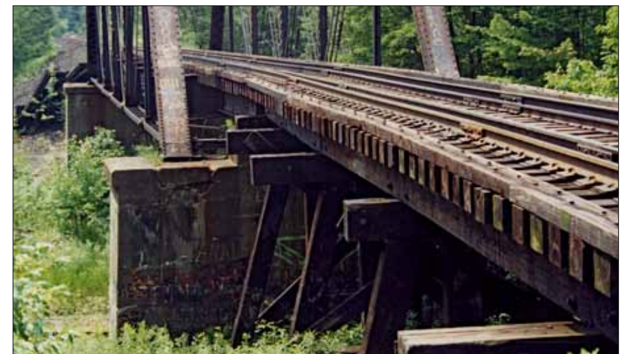
On the north end of the bridge, the tracks begin curving at the pier on which the bridge rests.
