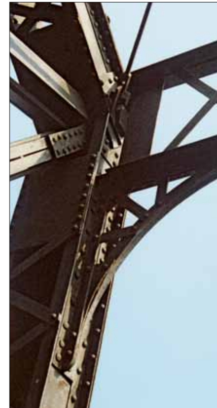
This photo looks up at joint U1 from inside the bridge and shows the anchor for the upper horizontal cross bracing (the X bracing visible above the engine in the lead photo).
