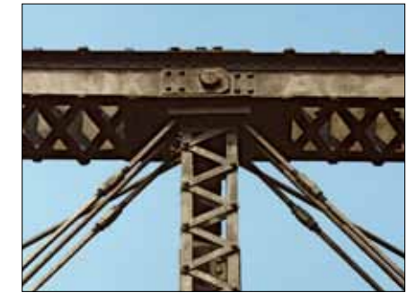
This photo of U3 shows the lattice bracing and how the tension rods and posts all join at a pin on the upper chord. Also note the solid turnbuckles.
