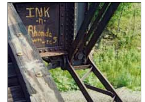
In contrast to the upper joint, this photo at L2 shows how the center rod terminates at a separate pin through the post rather than the common pin on the lower chord.
