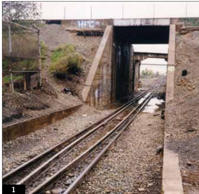
1 Looking north along the Union Pacific tracks through the levee, the Southern Pacific crosses over the UP on two tracks above. The wooden flood doors, hidden in the shadows, are on the other side of the embankment. Mark Bridgwater
